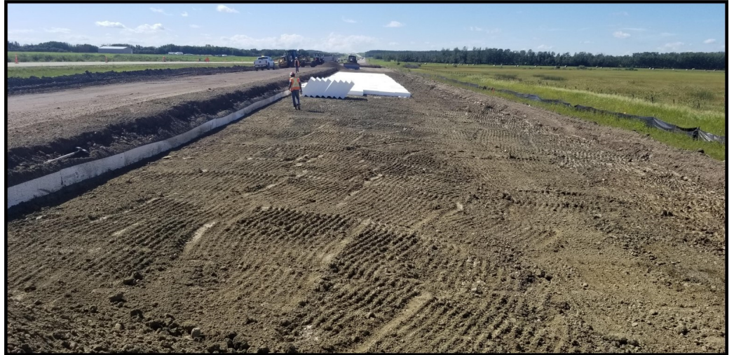
Highway 11 – Restoration of Ride Quality
